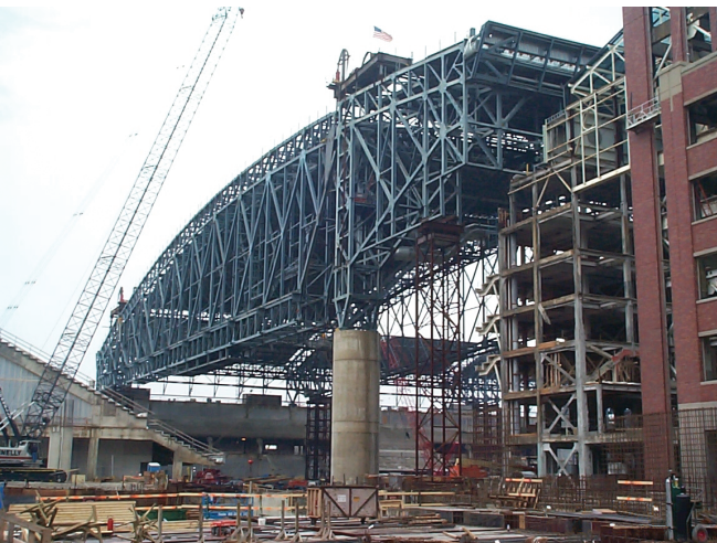
Fig. 6-1. Sequenced jacking of a suspended roof system at Ford Field, Detroit, MI (photo courtesy of SmithGroup).
