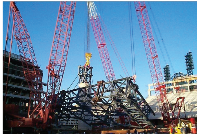
Fig. 6-2. Heavy assembly lifted from horizontal to vertical at Ford Field, Detroit, MI (photo by Ruby + Associates, Inc.).
